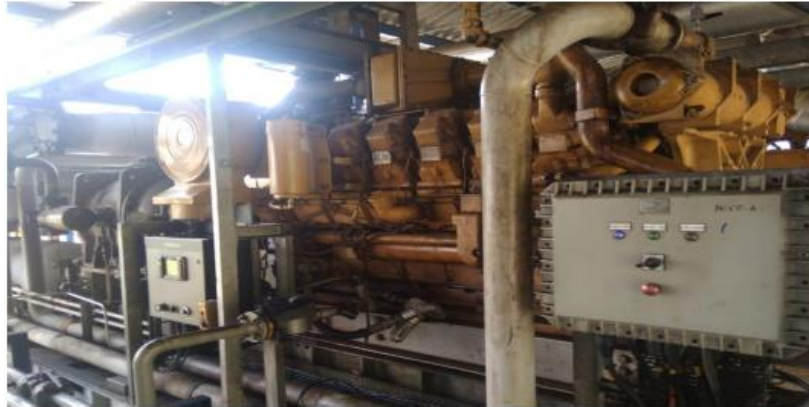
Gambar 1. Mesin austcold gas engine caterpillar
