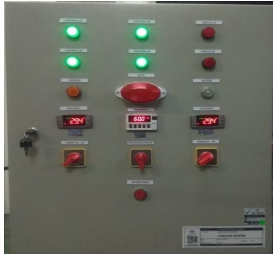
Gambar 5. Electrical panel control.
