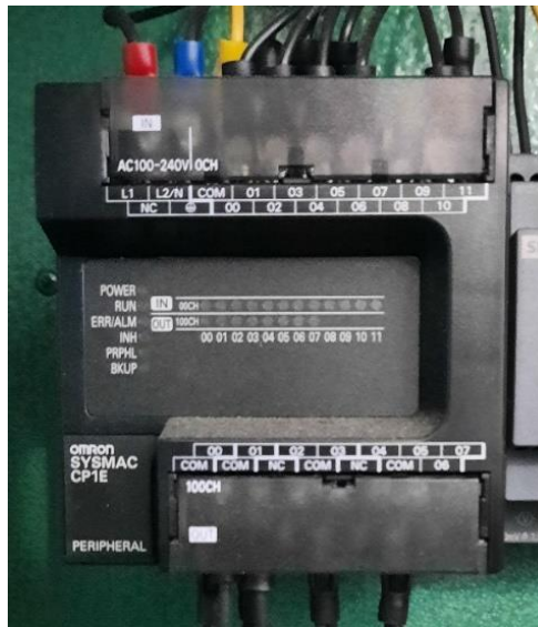
Gambar 5. Programmable Logic Control (PLC).
