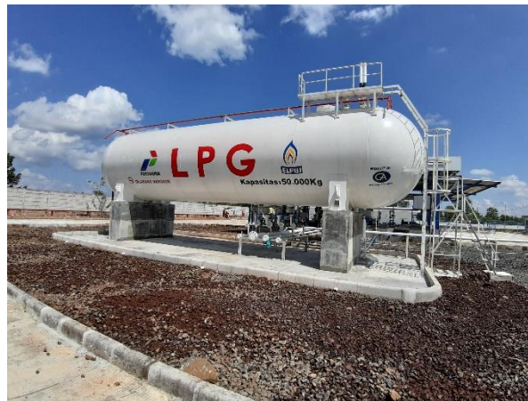
Gambar 1. LPG storage tank 50 T
