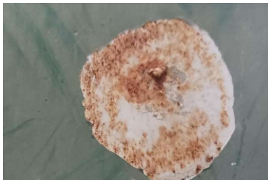
Figure 2. Uniform rust on the tank head
